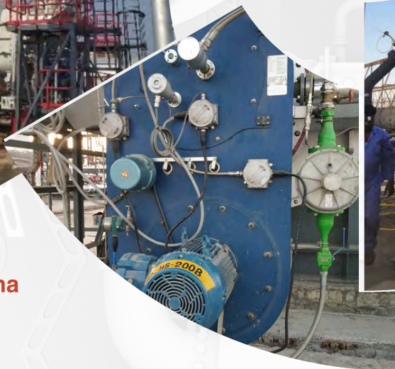
Heater Treater Mehsana field, ONGC (India)
